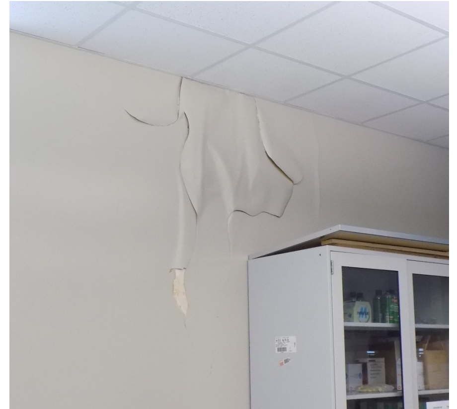
Water Damage to Walls from Roof Leaks
