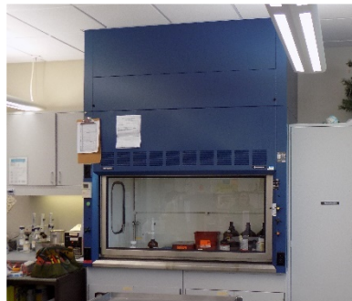
Chemical Fume Hoods
