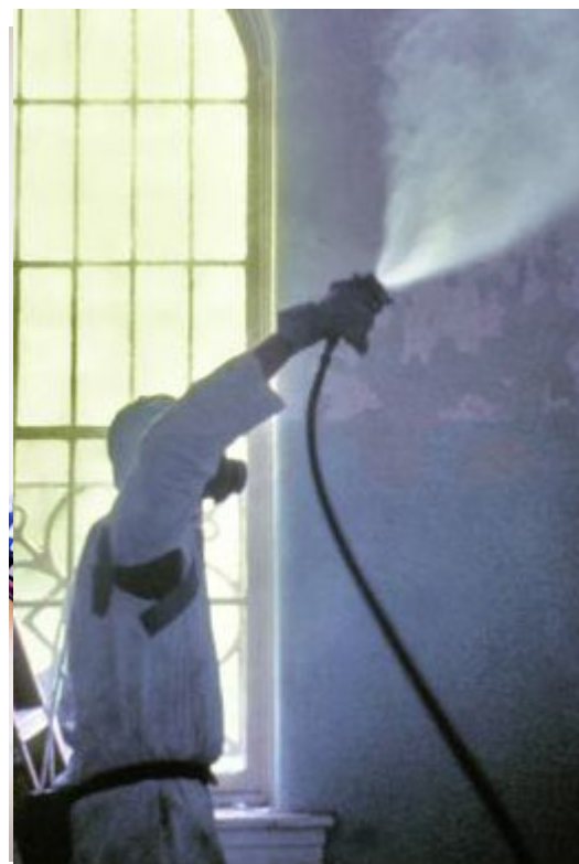
Worker wears protective mask and suit while preparing surface to avoid exposure to lead-based paint.
